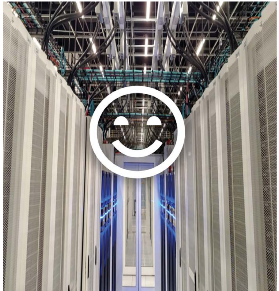
FIGURE 11: A completed and well-commissioned data center leads to both a happy data center and a happy client.
